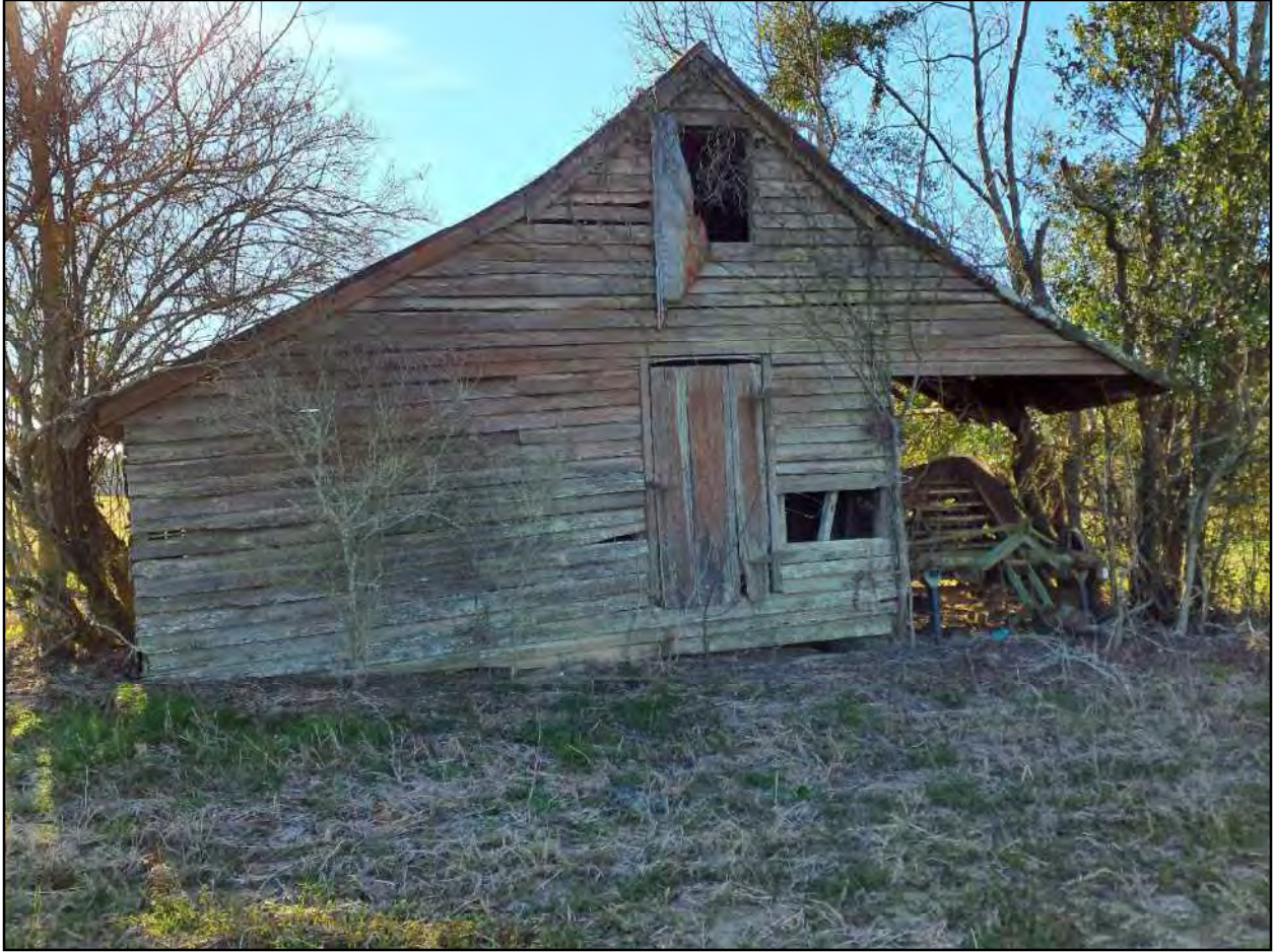
Figure 3.6 Abandoned wood plank structure at Locus 3 in Parcel 56 19 of the Heart Pine Solar project area.
