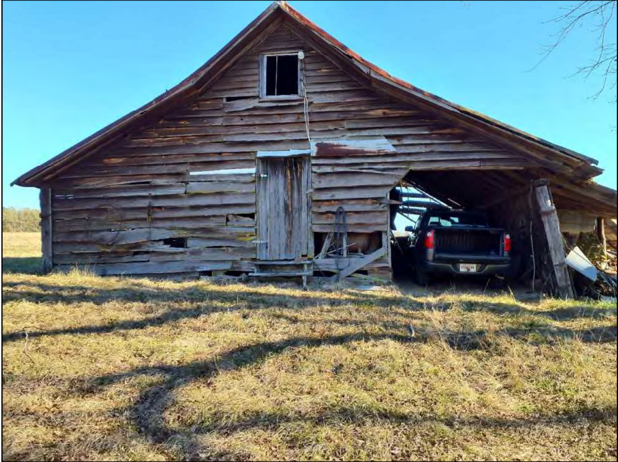
Figure 3.4 Wooden plank structure in use as vehicle/equipment storage facility at Locus 2 in Parcel 56 19 of the Heart Pine Solar project area.
